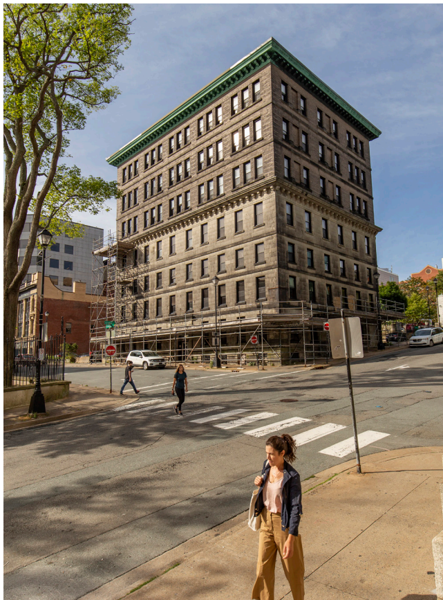
Fig. 17 Layers of site history are evident in the masonry changes on the exposed west wall of the Dennis Building
